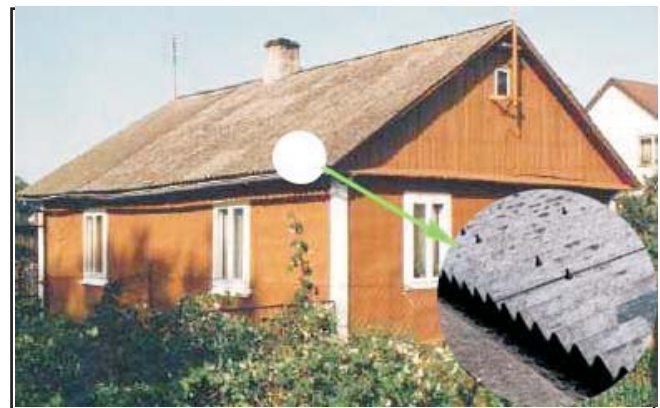
Asbestos roofing common for industrial and other sheds is risk-laden.
